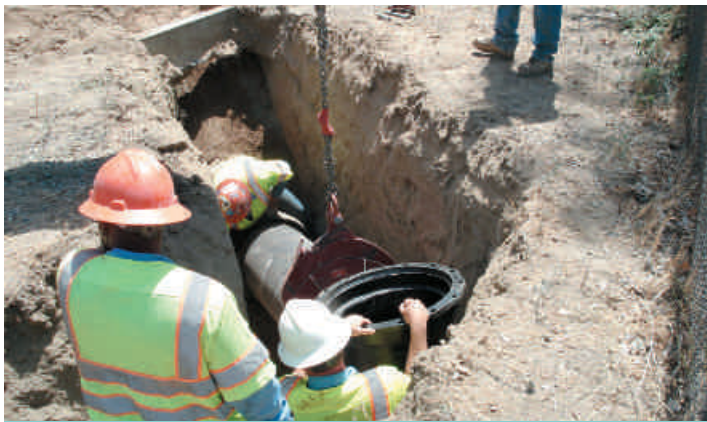
EVWD crews install 30-inch pipe along Sterling Avenue. The 6th Street Project will continue this pipeline an additional two miles to Plant 40.
